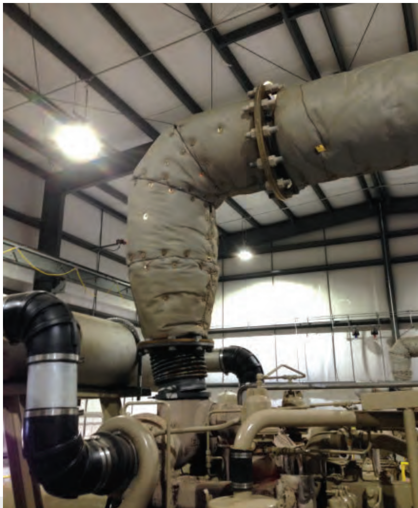
■ The failure of this expansion joint (left) located at the engine turbocharger exhaust flange resulted from inadequate support and excessive thermal growth of the long exhaust line (right) running from the engine to the catalyst outside the building wall.
