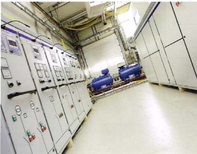
The automatic current controller had to be installed into the complete system
