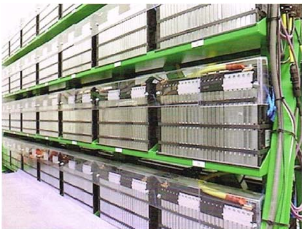
The batteries have to be treated well
