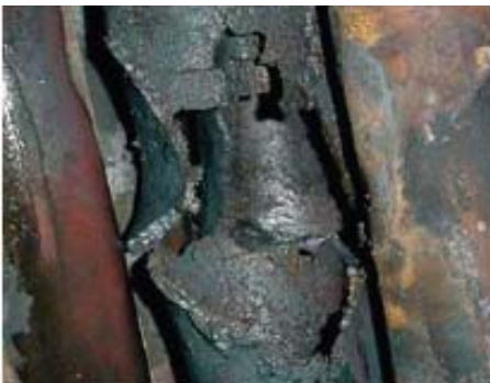
Tube burst due to short-term overheating
