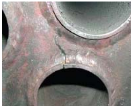
Creep cracks in a boiler end plate due to long-term overheating
